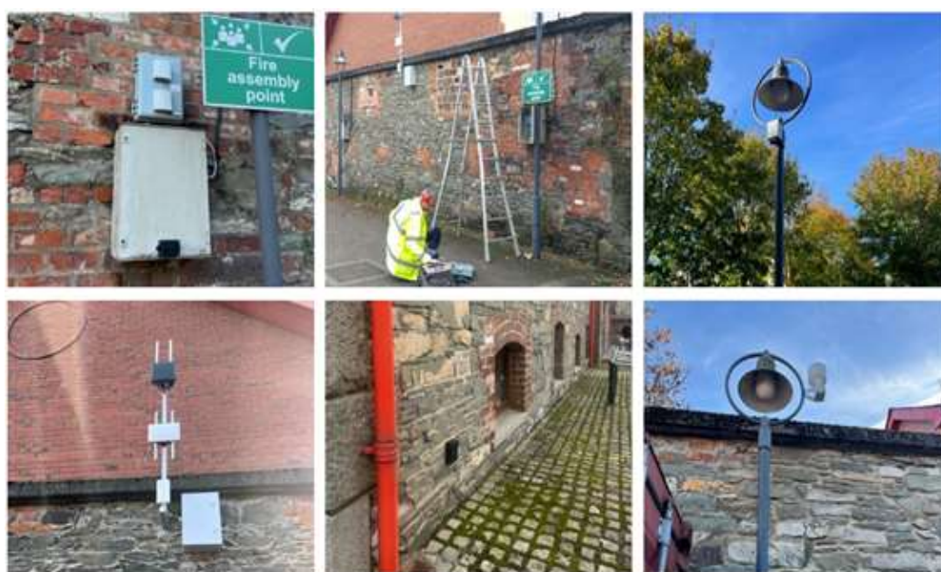
Figure 22: Dundalk (IE)- Installation of sensors
